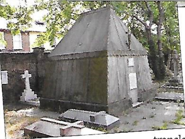
The mausoleum limewashed and gilded and (below) how it looked before the work started.
